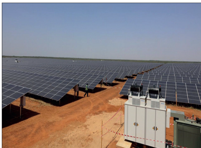
Photo 1: Bokhol photovoltaic power plant
