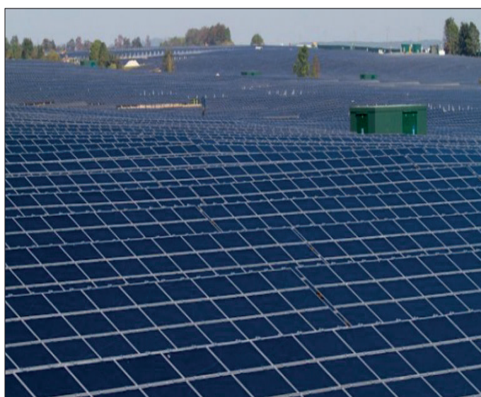
Photo 2: Malicounda solar power plant
