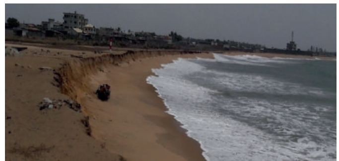
A) Before the work : Reference situation of the coast of the cross-border segment at Hillacondji in Benin
